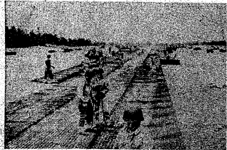
AVIATION ENGINEERS . . . Constructing a mat runway on Siapan during World War II.
