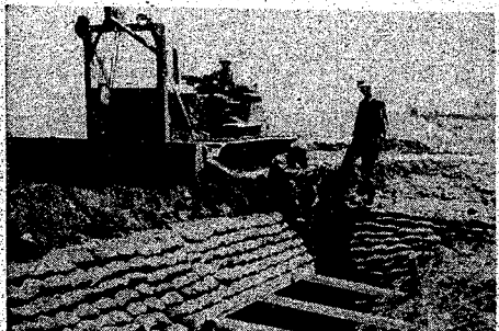
KOREAN ENDEAVOR . . . Road construction in Korea proved to be a major task for the engineers.
